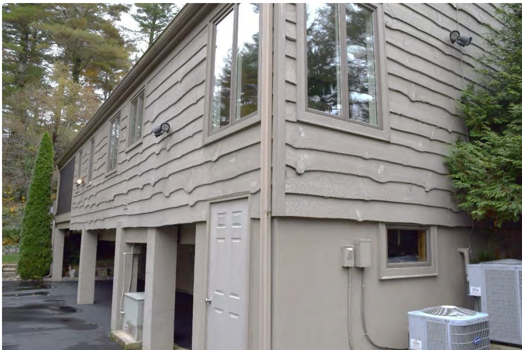
Anders House, South and Rear Additions, Side (South) and Rear (West) Elevations, Looking Northeast.
